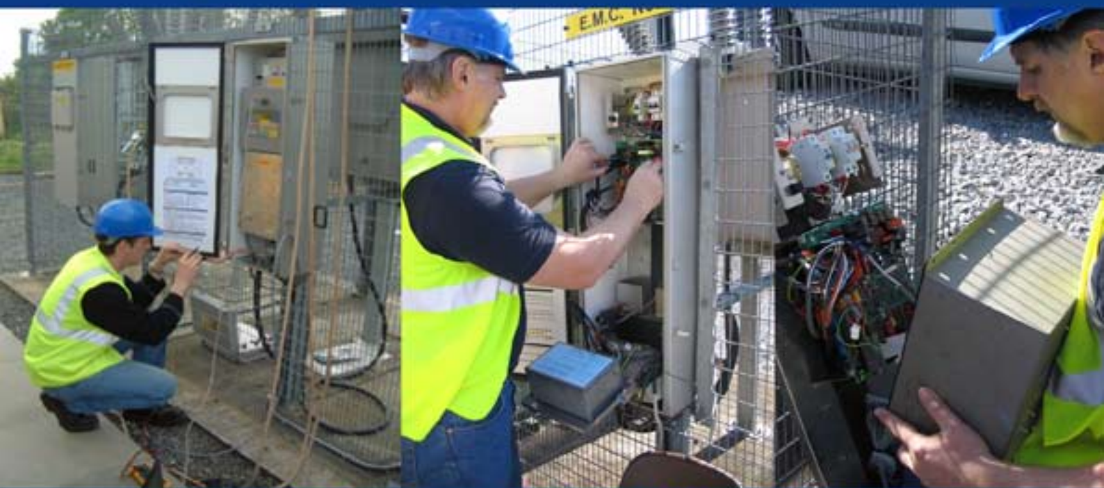
Above: Renley Service Engineer inspecting Control Cubicle and Umbilical cable connections, on a substation mounted recloser. Another Renley Service Engineer is performing a Capm2 to Capm5 upgrade.
